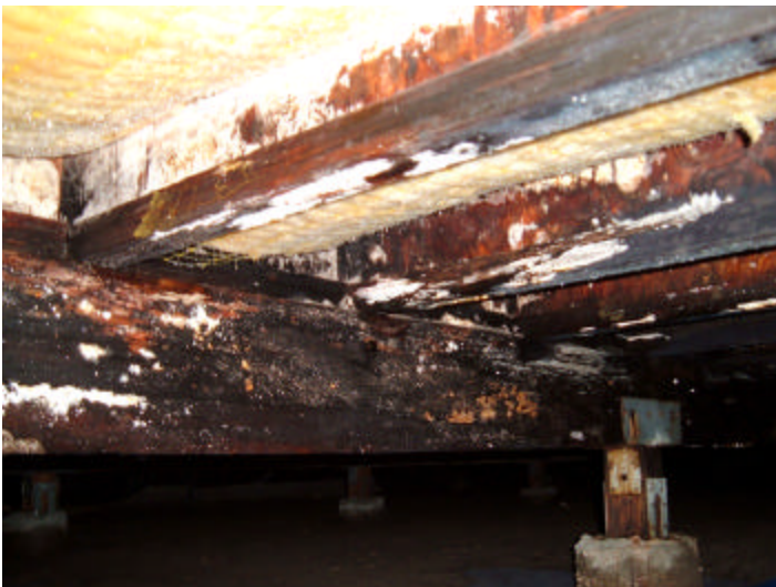
Above: Damage found in the crawlspace of a home less than seven-years old.
